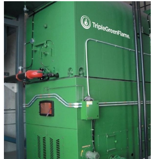
Figure 28: Installed biomass boiler available from Triple Green Products (TGF 2020).
