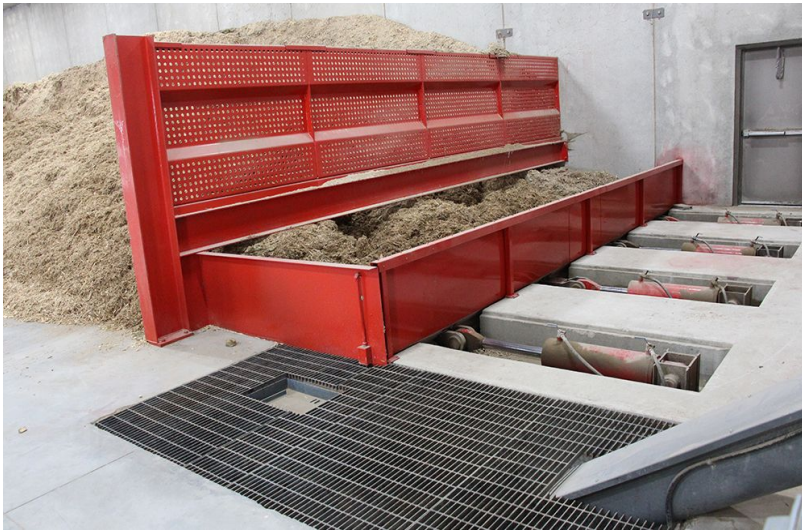
Figure 27: Walking floor moving biomass feed into augers feeding a biomass heating system (TGF 2020).
